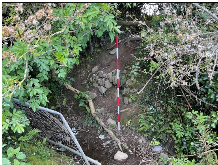
Plate 12 Bank on northern boundar of F3
